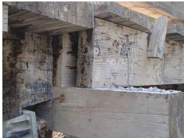
Figure 1-24: Span 5, girder 1 leaning outwards.
