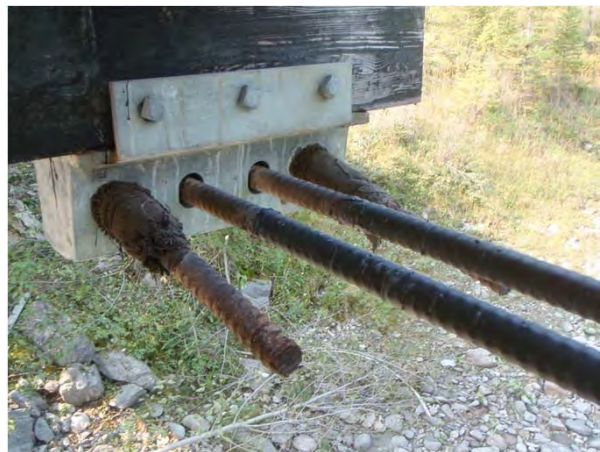
Figure 1-16: Typical dywidag bars.
