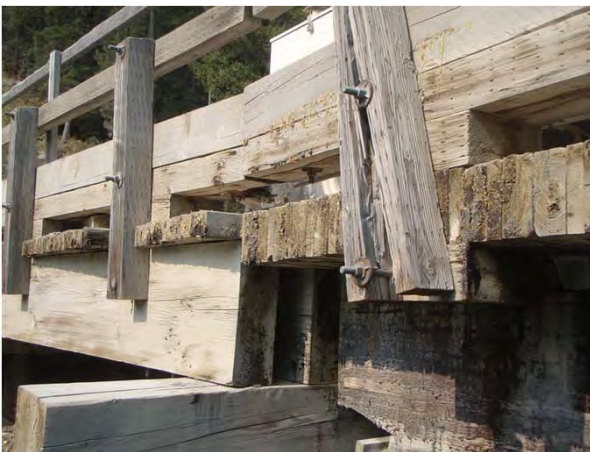
Figure 1-9: Damaged railing post.
