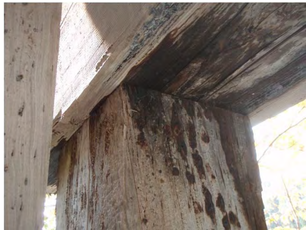
Figure 1-18: Pier 1 cap crushing at upstream column.
